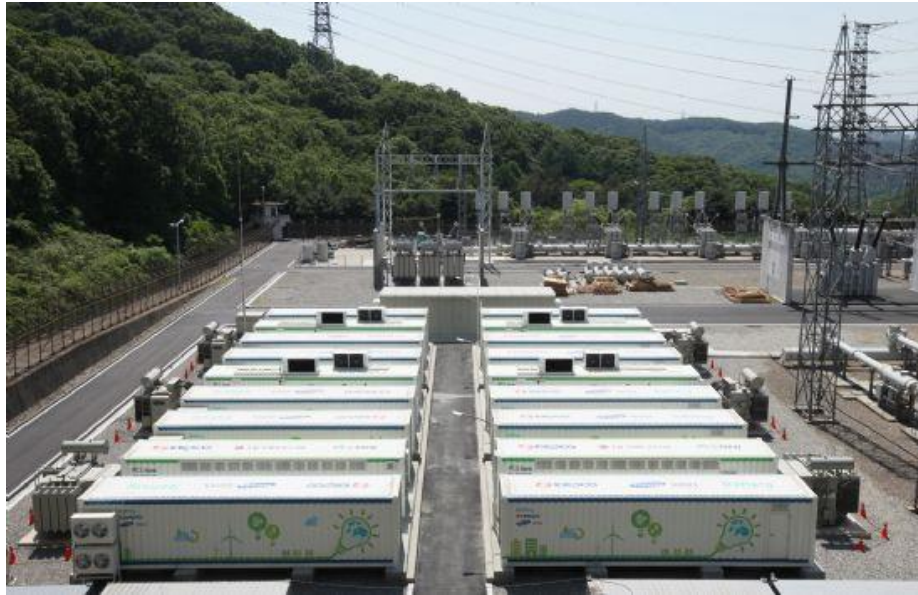
Engineering by KEPCO
